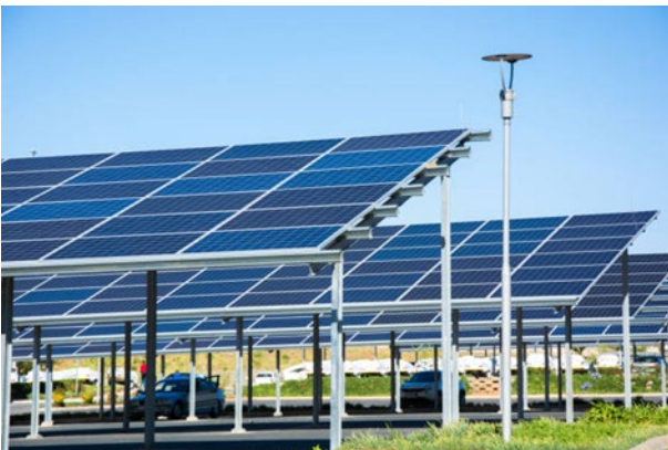
Figure 4-7 Carpark Shade Structure Mounted Solar Panels Angled Southwards
